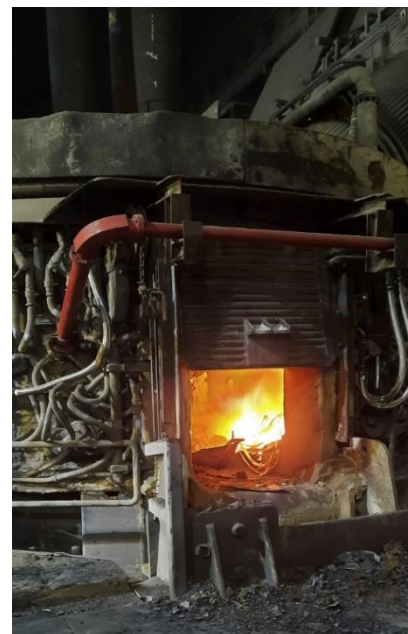
Flame of the new burner using the AM
